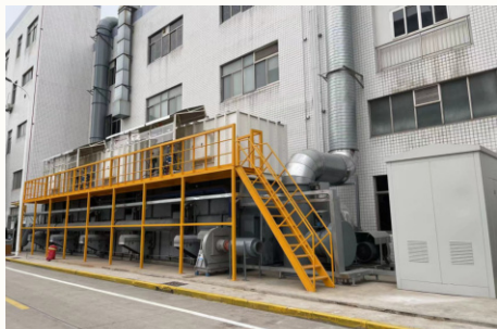
Spraying Waste Gas Disposing Facility
