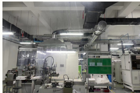
Waste Gas Disposing Facility in the Sample Making Workshop
